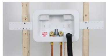
RIGHT DRAIN, BOX MOUNTED CENTER
