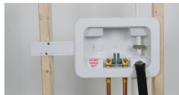
RIGHT DRAIN, BOX MOUNTED ON RIGHT STUD WITH SECONDARY DRAIN LINE
